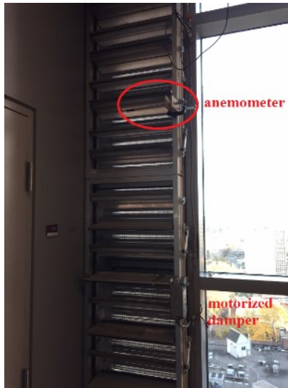
Figure 3: Natural ventilation velocity measurement near inlet dampers.
