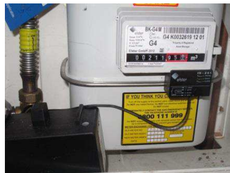
Figure 1. Gas monitoring equipment installed by SMS solutions
