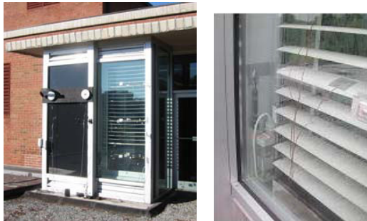
Figure 2 Smart façade system installed in the College of Architecture Building, Georgia Institute of Technology, Atlanta, GA, U.S.A.
