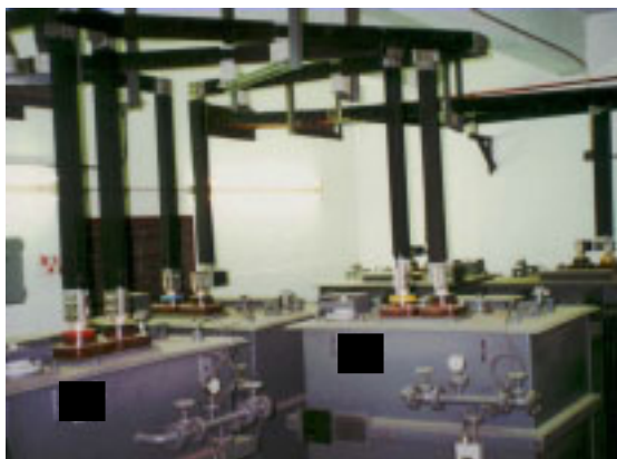
Fig 3 Transformer Room under the office floor
